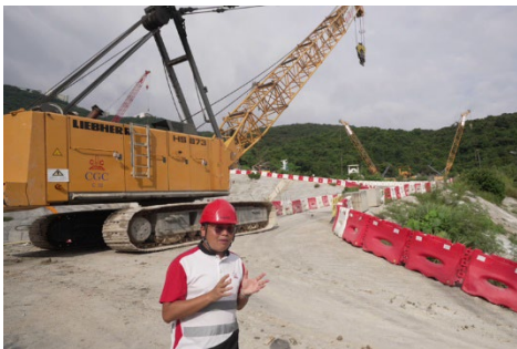
LHK_HS873_Transform_after.png German Leung of China Geo-Engineering Corporation on site with the transformed HS 873 HD.
