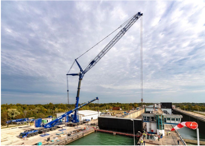
liebherr-ltm-1650-8-1-&-ltm-1450-8-1-msg-01.jpg Almost at its destination: the 84-tonne lock gate is lowered into the chamber.
