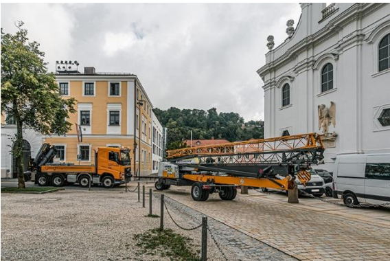
liebherr-l1-24-beuthauser-passau-dom-05.jpg Its tight turning radius proved an advantage for the L1 en route.
