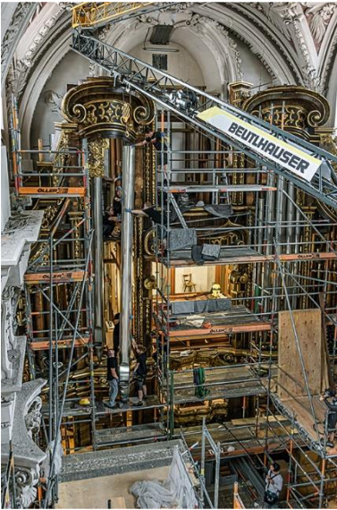
liebherr-l1-24-beuthauser-passau-dom-03.jpg The metres-long pipes are lowered into the nave one by one.
