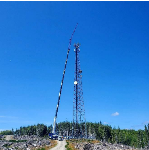
liebherr-Snell-Crane-Working-2.jpg The LTM 1120-4.1 performs work on a 250 ft. cell tower with a 23 ft. extension with offset.
