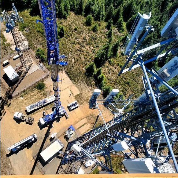
liebherr-Snell-Crane-Working.jpg Snell Crane Service utilizes their LTM 1120-4.1 to perform work on a cell tower.
