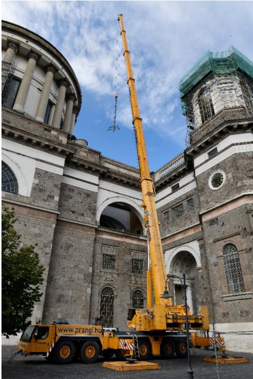
lwe-ltm-1250-6-1-prangl-esztergom-1.jpg A Liebherr LTM 1250-6.1 from Prangl on site in front of the cathedral in Esztergom.
