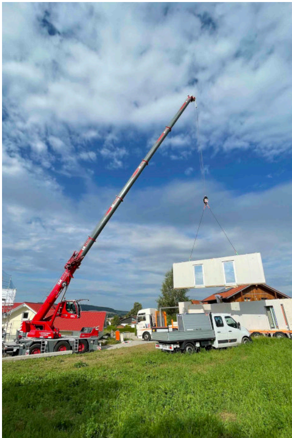
liebherr-ltc1050-3-1-leitl-2.jpg Leitl uses the LTC 1050-3.1 for its first job erecting a prefabricated house.
