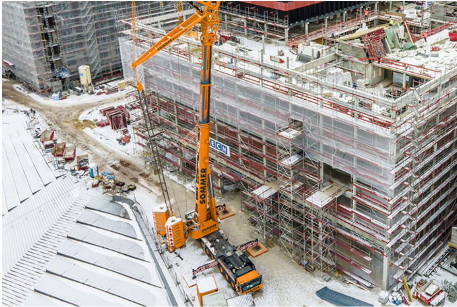
liebherr-ltm1450-8-1-sommer-04.jpg VarioBallast® on the LTM 1450-8.1 is worth its weight in gold on constricted sites.
