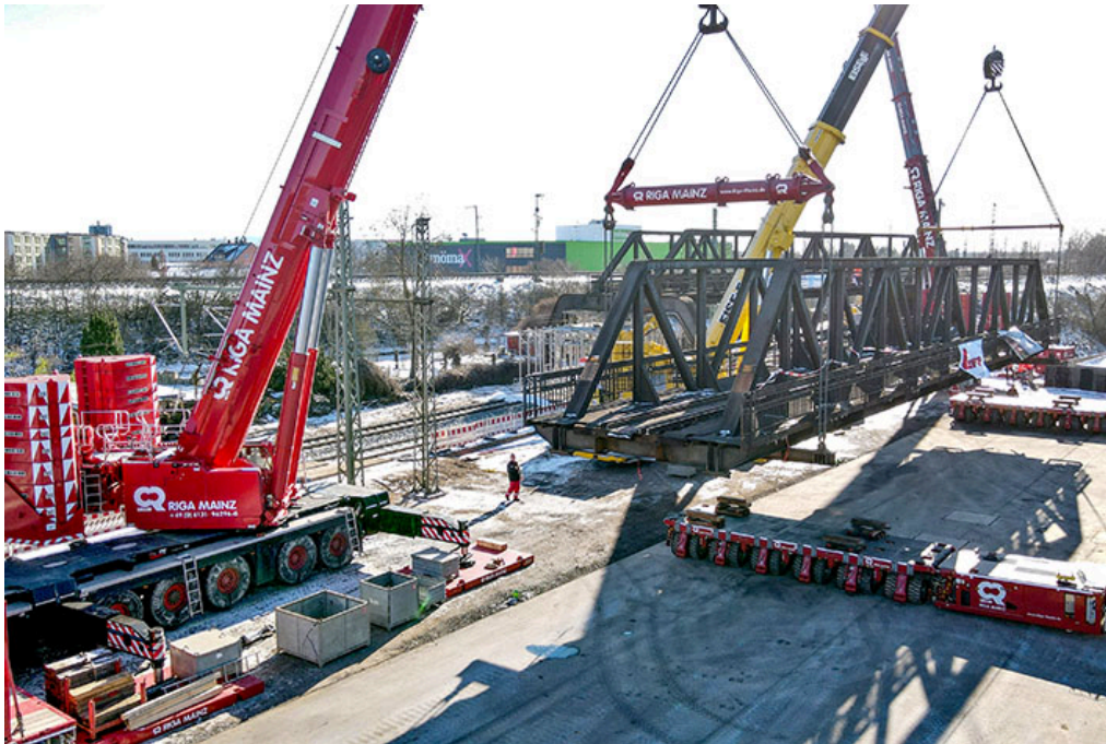
liebherr-riga-ltm1650-8.1-eisele-ltm-1500-8.1-motive03.jpg Heavy duty modules – 6-axle SPMTs transport the historic bridges to the refurbishment site.
