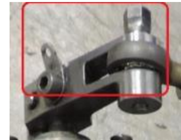
Retaining cable missing
