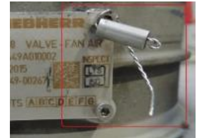
Lock wire or seal damaged
