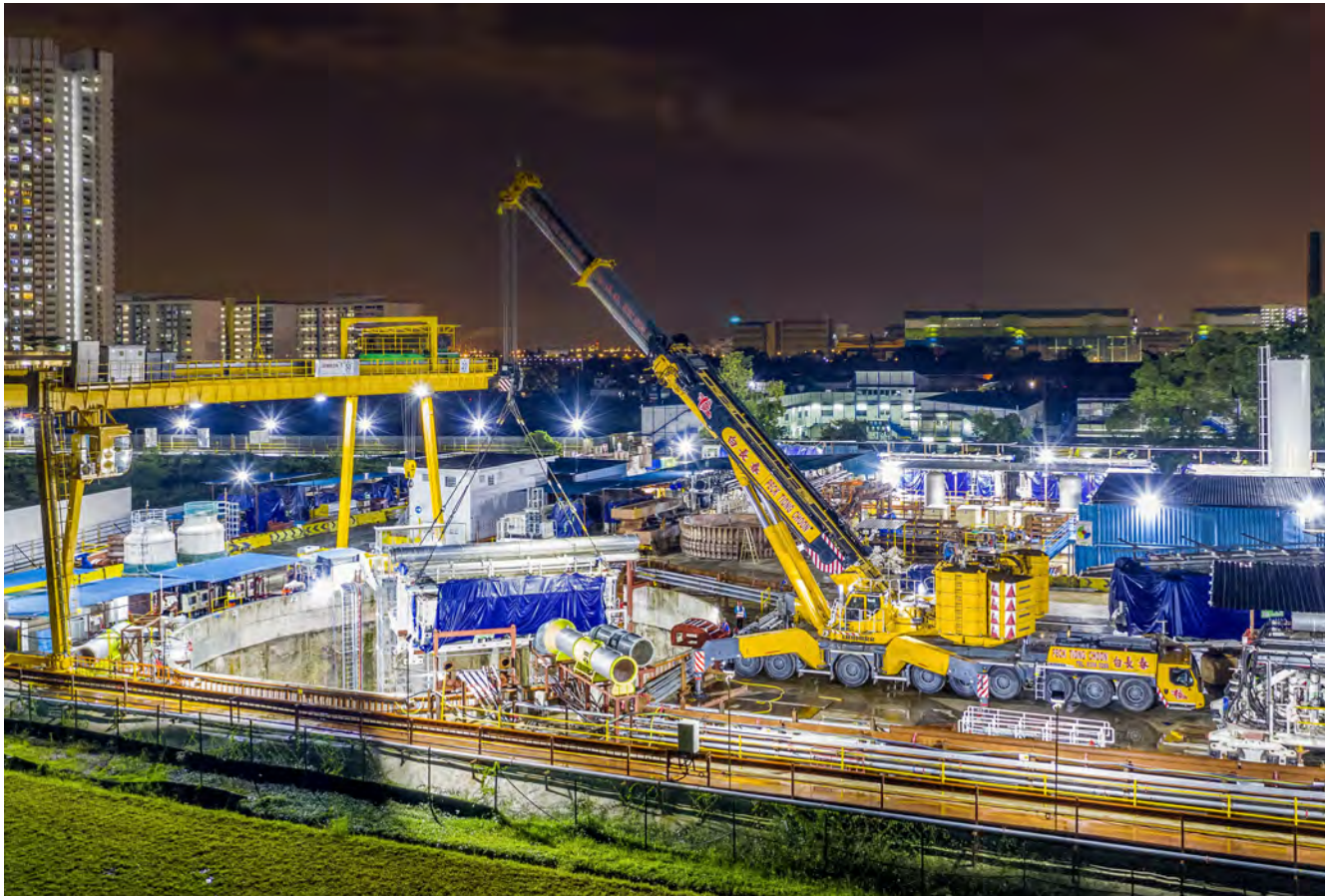
Night shift – an LTM 1750-9.1 setting up a site for a massive tunnel project in the mega city, which is designed to collect the rainwater from the metropolis at a depth of 60 metres. Peck Tiong Choon Leasing operates 16 Liebherr cranes in Singapore.
