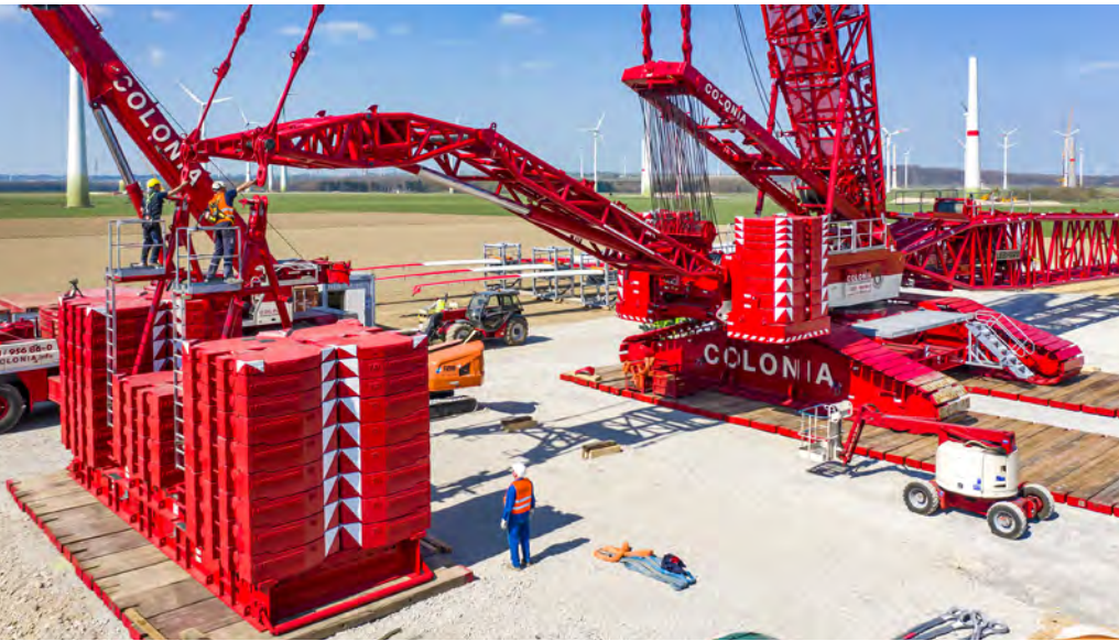
Heavy duty – 400 tonnes of suspended ballast are attached to the folding frame known as the “V-Frame”.
