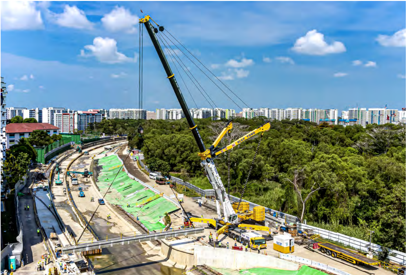
The most powerful Liebherr mobile crane in Singapore too – massive reinforced concrete beams on the hook of the Hiap Tong Corporation's LTM 11200-9.1.
