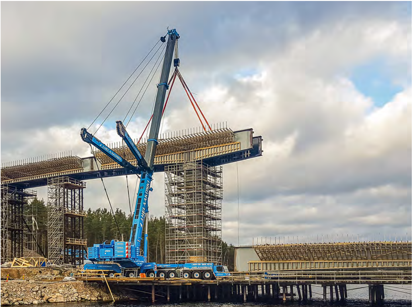
Bridge building in Finland – Helaakoski’s “new” LTM 1750-9.1 also came from Liebherr’s pool of used cranes. The freshly resprayed nine-axle machine has been in action for several months – and is actually the most powerful mobile crane in the country.
