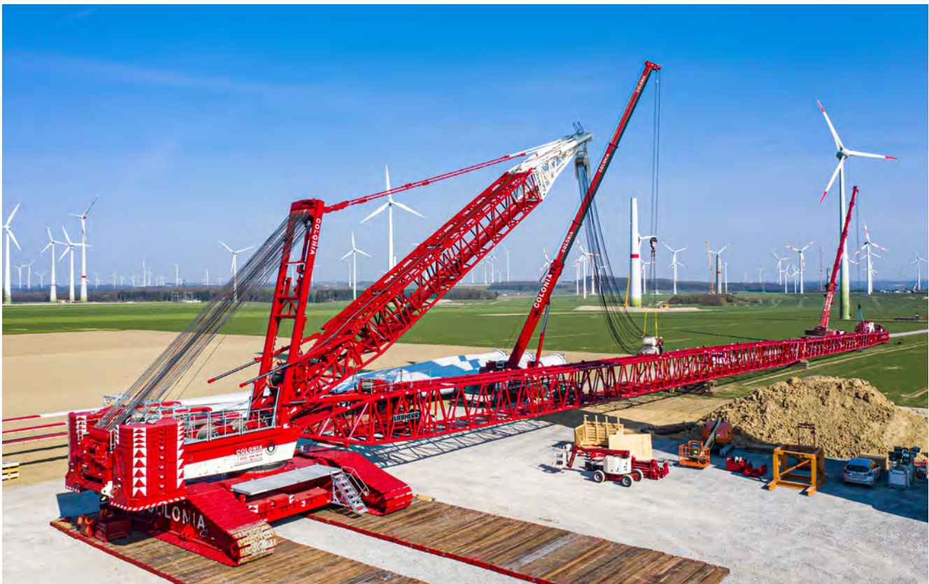
Two Liebherr mobile cranes were used for the set-up work. Here you can see the adjustment block for the derrick guying being positioned whilst the main boom is being assembled at the rear right.
