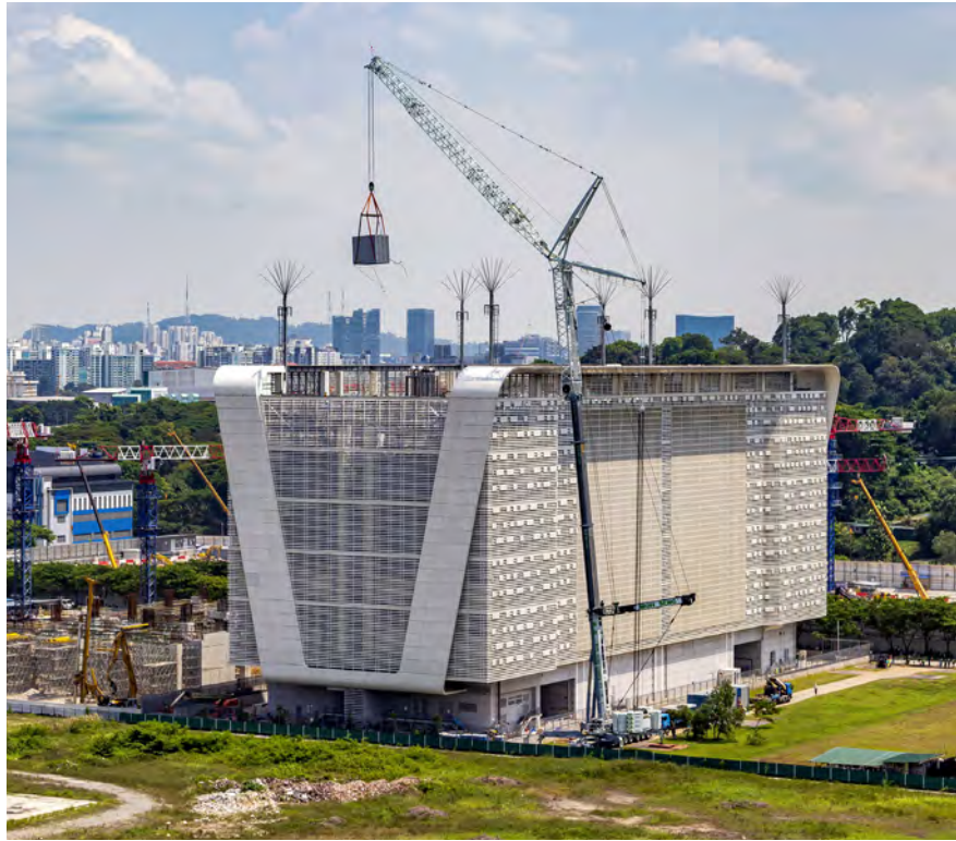
Modern metropolis – the LTM 1750-9.1 from Moh Seng Cranes hoists air conditioning units onto an industrial building.
