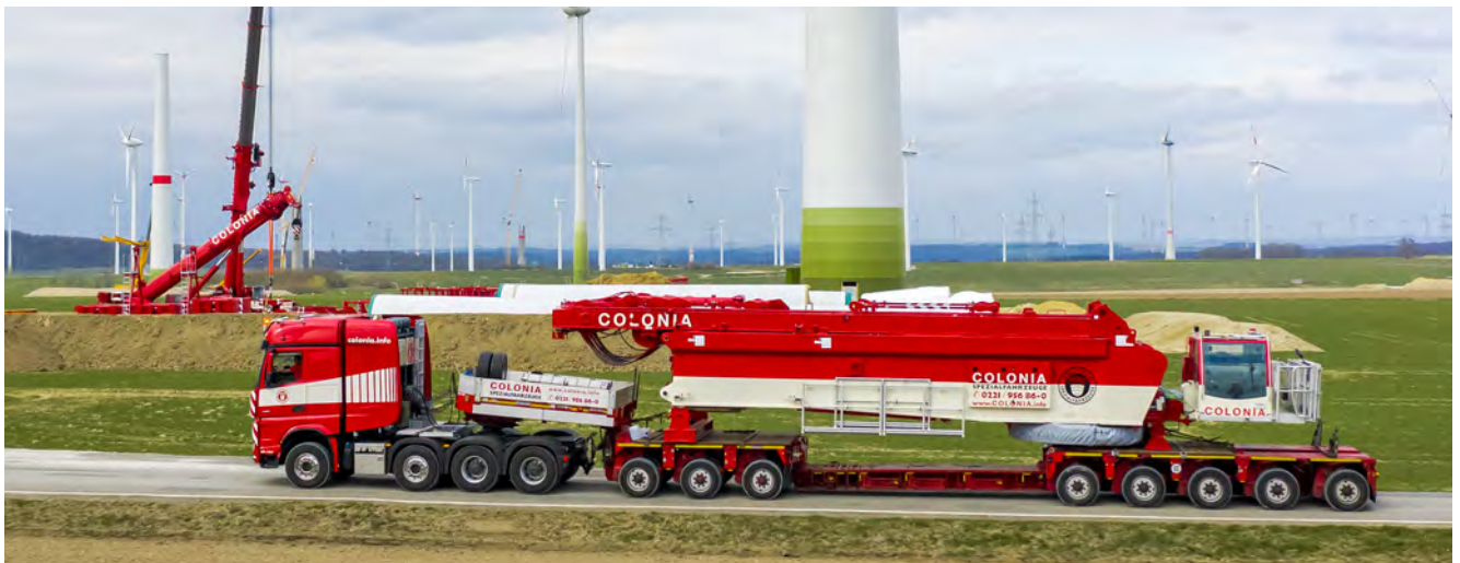
Slimline – the basic machine is designed to have a transport width of just three metres. Here you can see the superstructure of Colonia Spezialfahrzeuge's new LR 1800-1.0 arriving on site at the wind farm.
