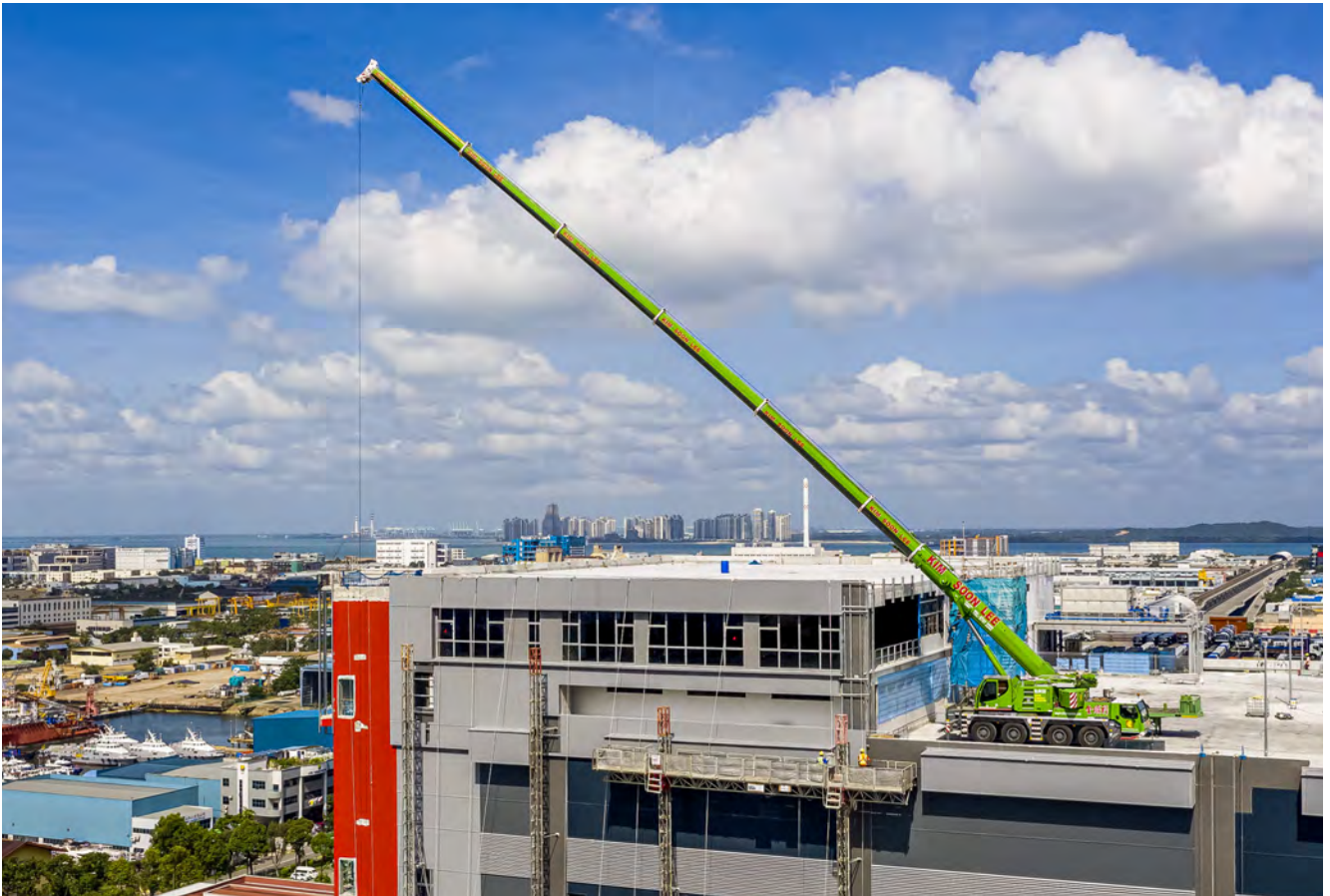
Fantastic view – an LTM 1100-4.2 the ready to install an external staircase on the flat roof of the building. The green crane belongs to Kim Soon Lee.
