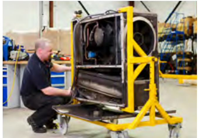
Maintenance of an HVAC system
