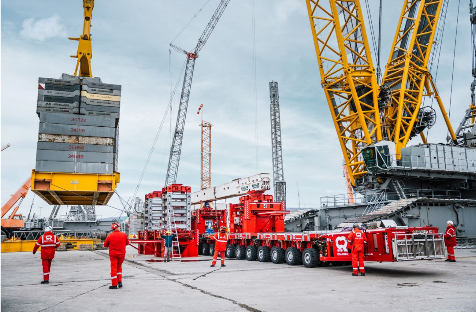
Five power lift towers and a 22-axle SPMT stand ready for a static load test.
