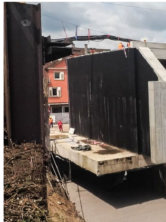
PLTs on SPMTs move prefabricated bridge components weighing up to 1850 tonnes to their final position in their first job.
