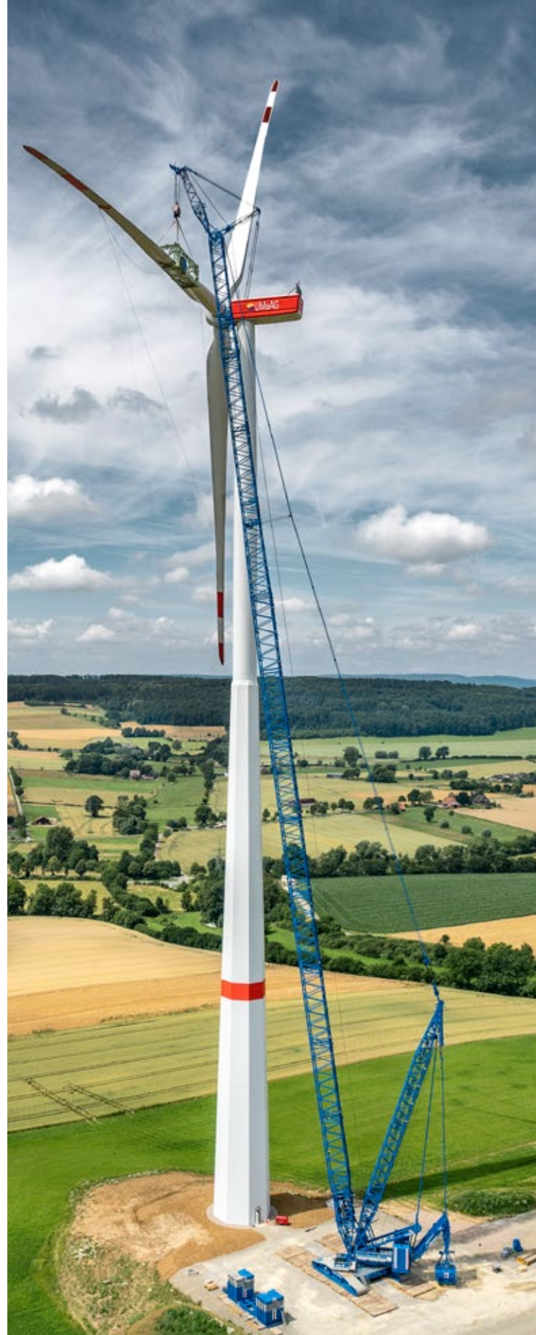
A LR 1700-1.0 used for the erection of a wind turbine in Germany
