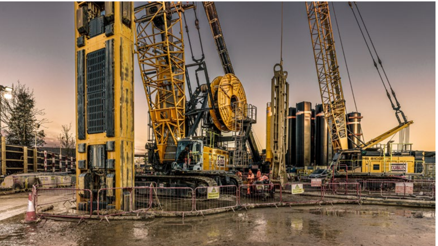
HS 8130 with slurry wall cutter and HS 8100 with slurry wall grab operating in London
