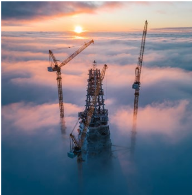
HC-L tower cranes used in the construction of Europe's tallest building, the Lakhta Tower in St Petersburg (Russia)
