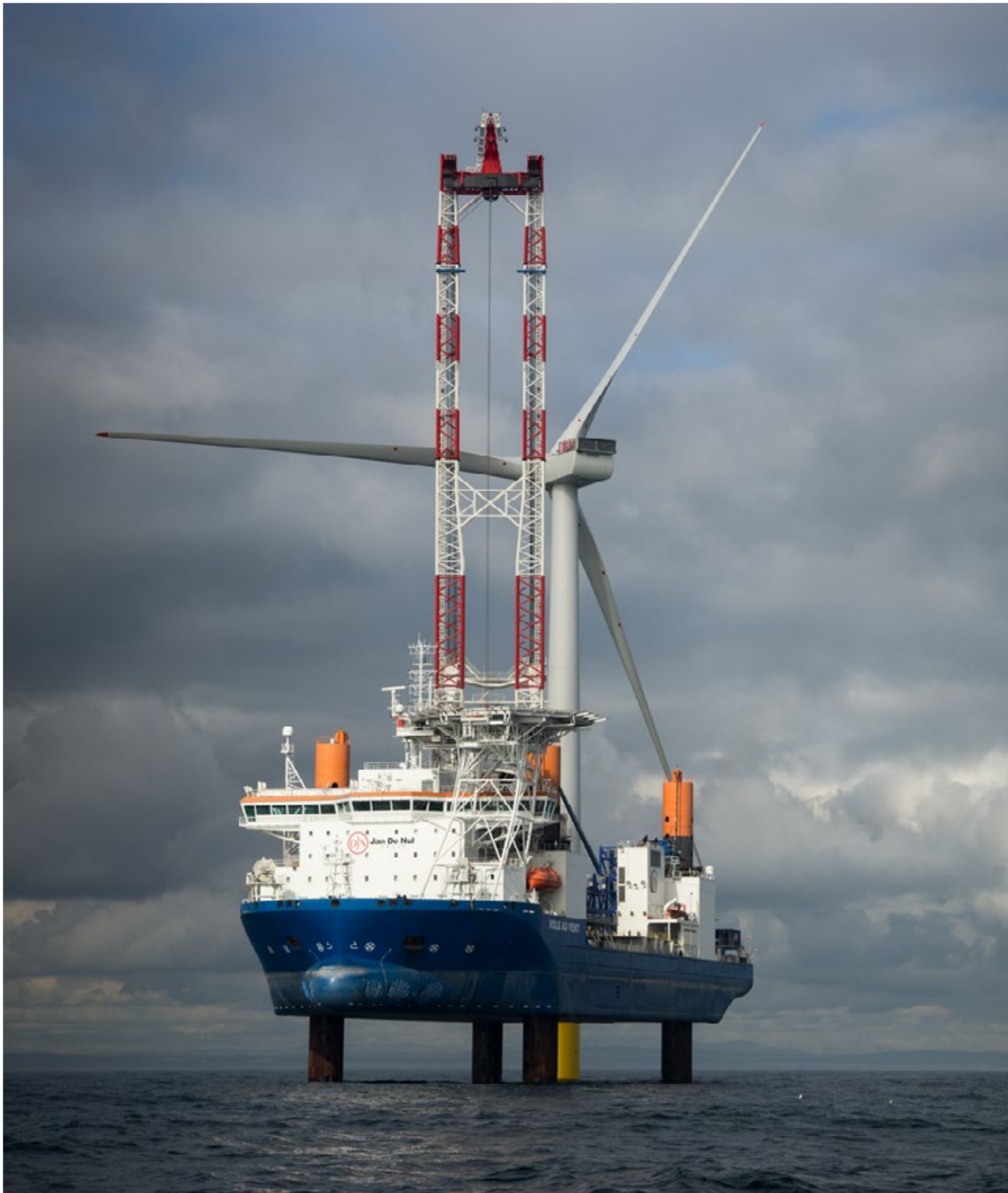
This crane around the leg CAL 45000, in operation on-board the "Vole au Vent", can lift up to 1,200 tonnes
