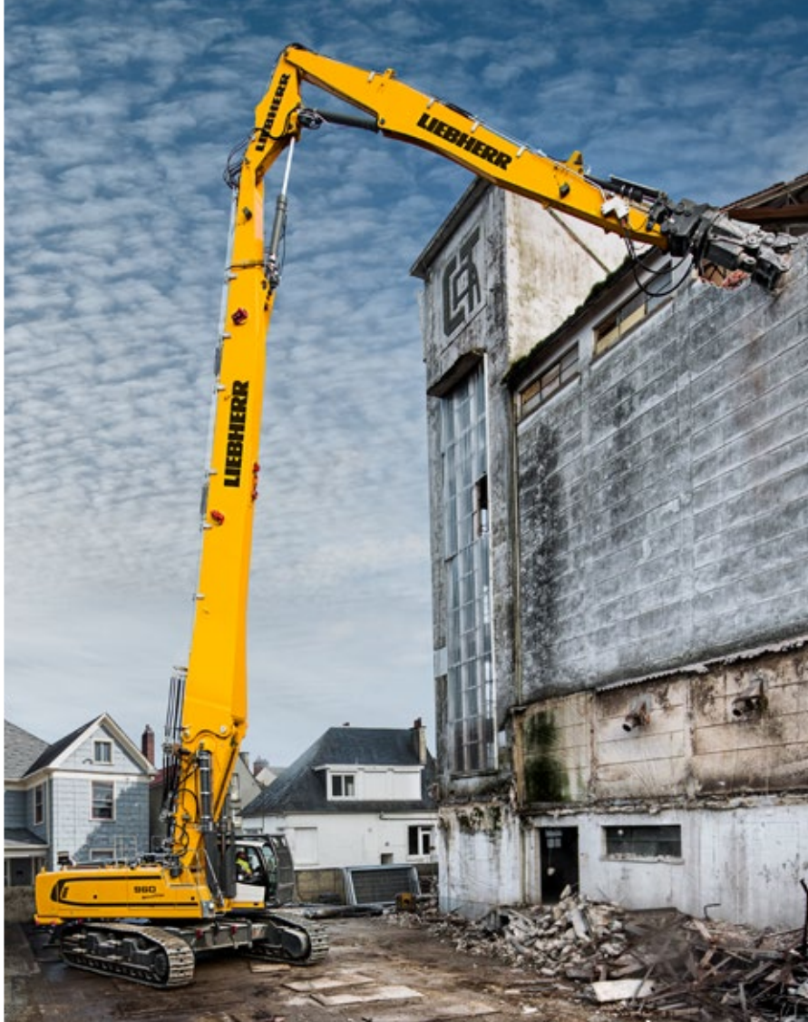
The crawler excavator R 960 used for the demolition of a silo in Frévent (France)
