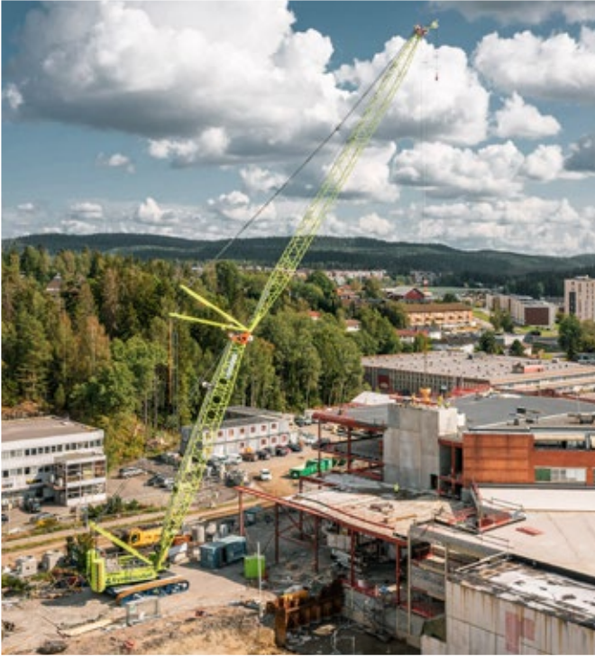
The battery-powered crawler crane LR 1250.1 unplugged used for lifting work in Oslo (Norway)
