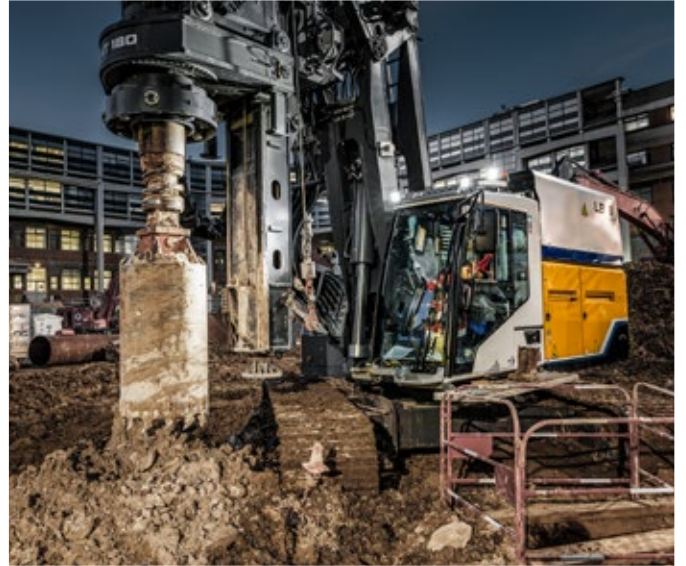
The battery-powered drilling rig LB 16 unplugged used for drilling work in Paris
