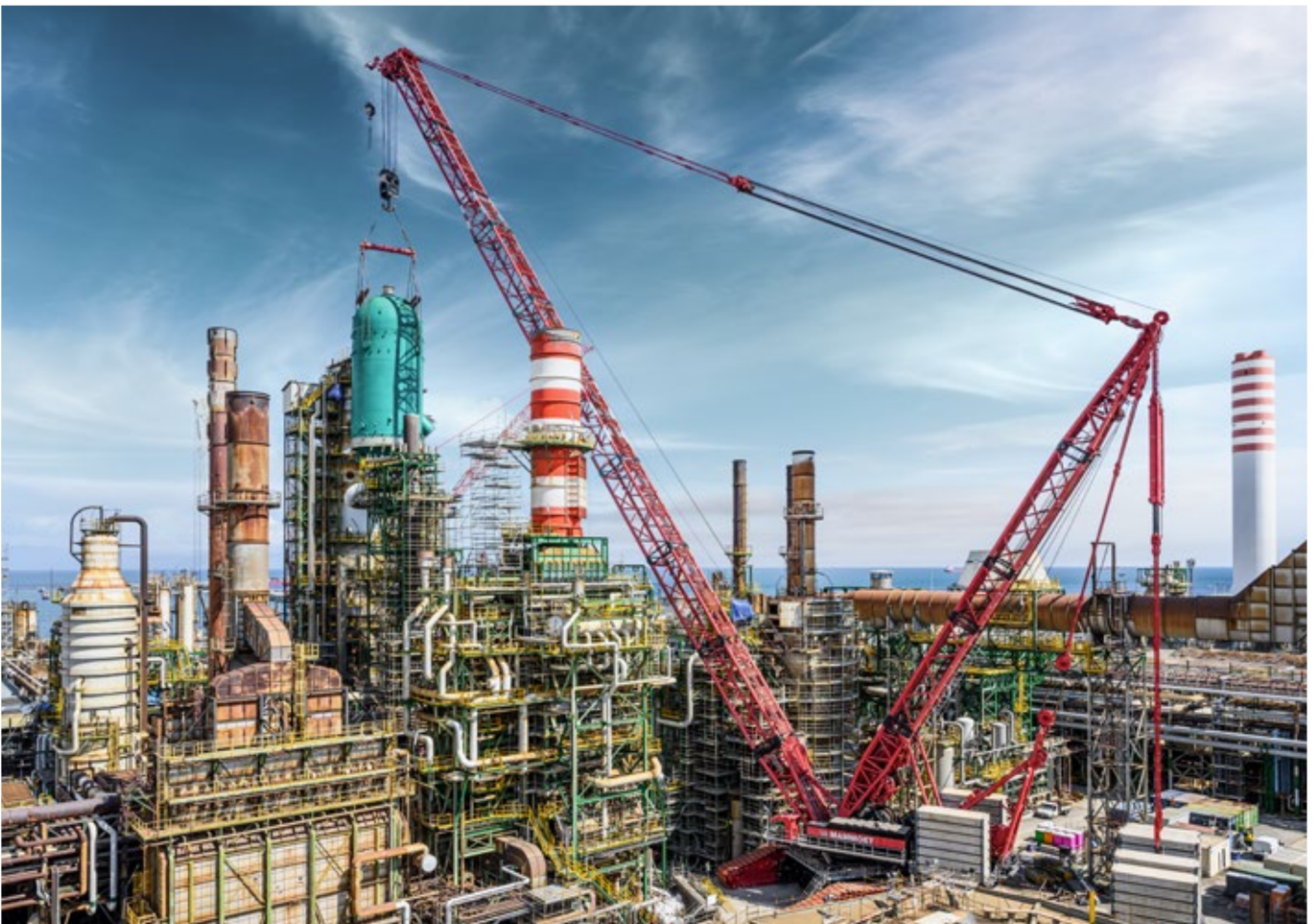
The LR 13000, the largest Liebherr crawler crane, at a petrochemical application in Italy
