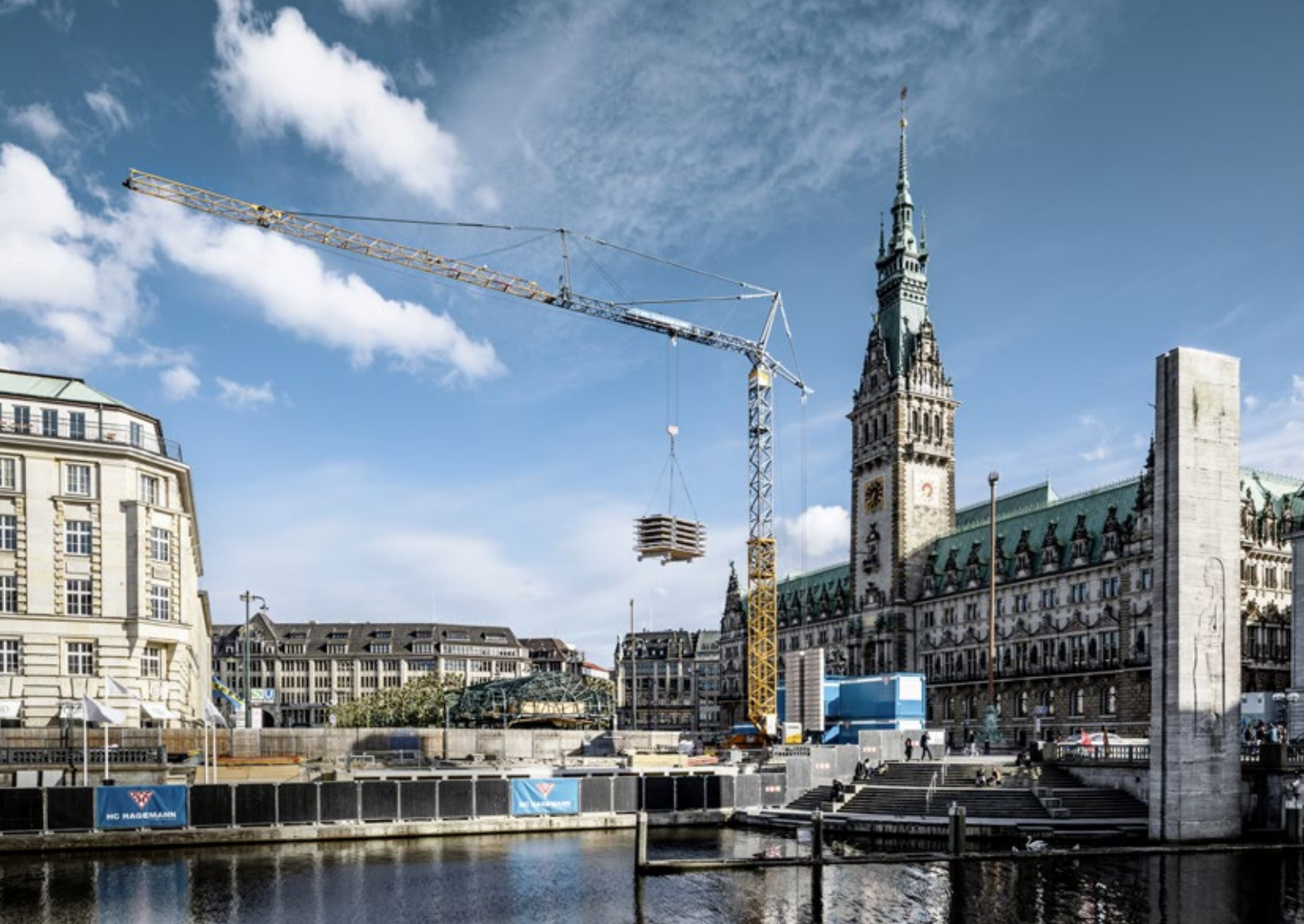
The fast-erecting crane 81 K.1 with increased load capacity at the Hamburg City Hall (Germany)
