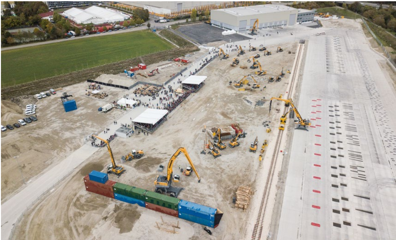
The new development and demonstration centre in Kirchdorf an der Iller (Germany)
