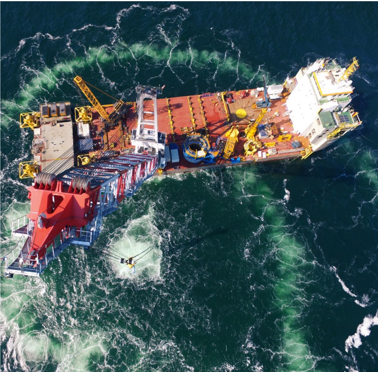
An offshore crane, type BOS 35000, installs a wind farm in the Baltic Sea
