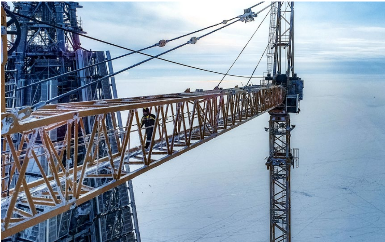
A Liebherr service technician maintaining a tower crane at the Lakhta Center in St. Petersburg (Russia), the tallest building in Europe
