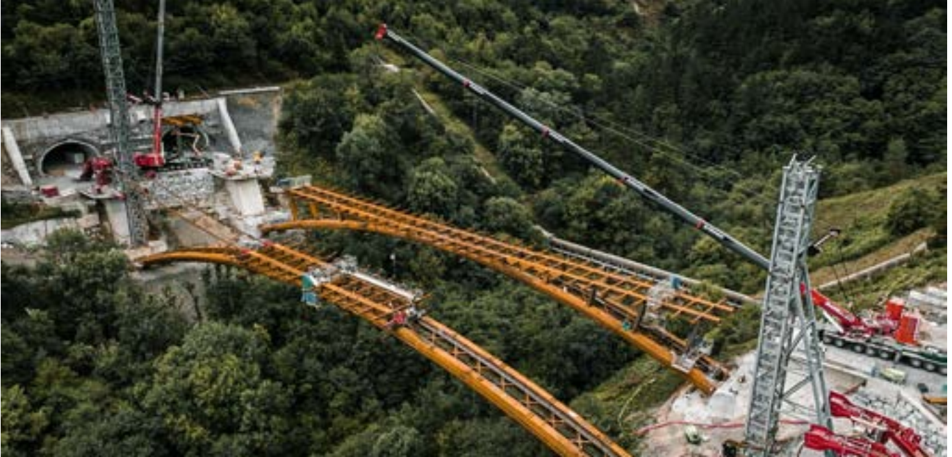
With its long boom, the LTM 1650-8.1 reaches over the valley with heavy steel components on its hook to hoist them precisely onto the viaduct.
