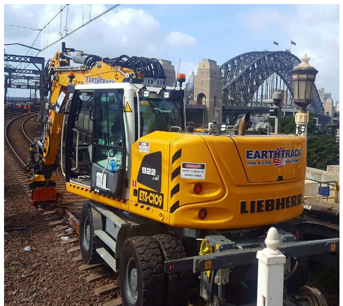
Earthtrack Solutions' A 922 Railroader working on the rail lines at Sydney Harbour Bridge.
