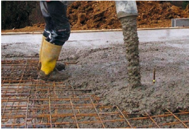
Flawless insertion of the concrete due to consistent concrete flow without deflections at the end of the hose.
