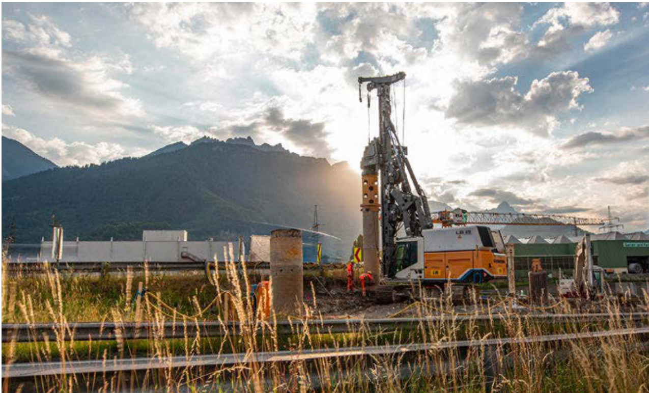
The first battery-powered drilling rig in the world, the LB 16 unplugged, is used on one of the largest roadwork sites in Western Austria
