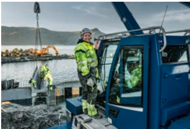
Site visit Mads Indresøvdde, Managing Director of Sunnmøre Kranservice AS, visits his new LTM 1110-5.2 at the shipyard. The company’s fleet of Liebherr cranes also includes a 250-tonne mobile crane and a brand new LTM 1060-3.1.
