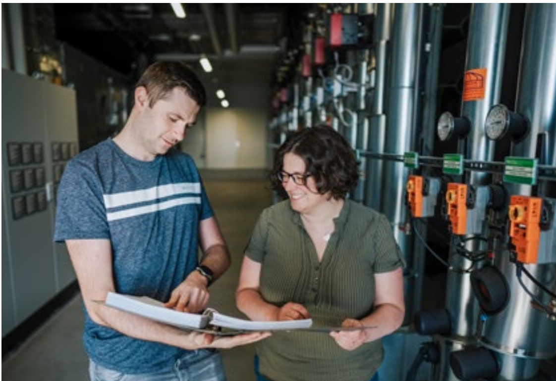
Christian Wölfle and Sophie Gantert check the heat flow meters on the canteen's heating manifold.
