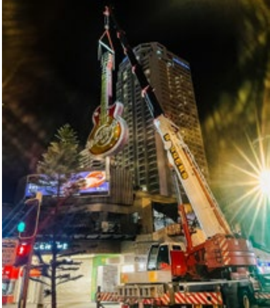
The LTM 1060-3.1 lifts the Les Paul guitar from the roof of the Hard Rock Café...
