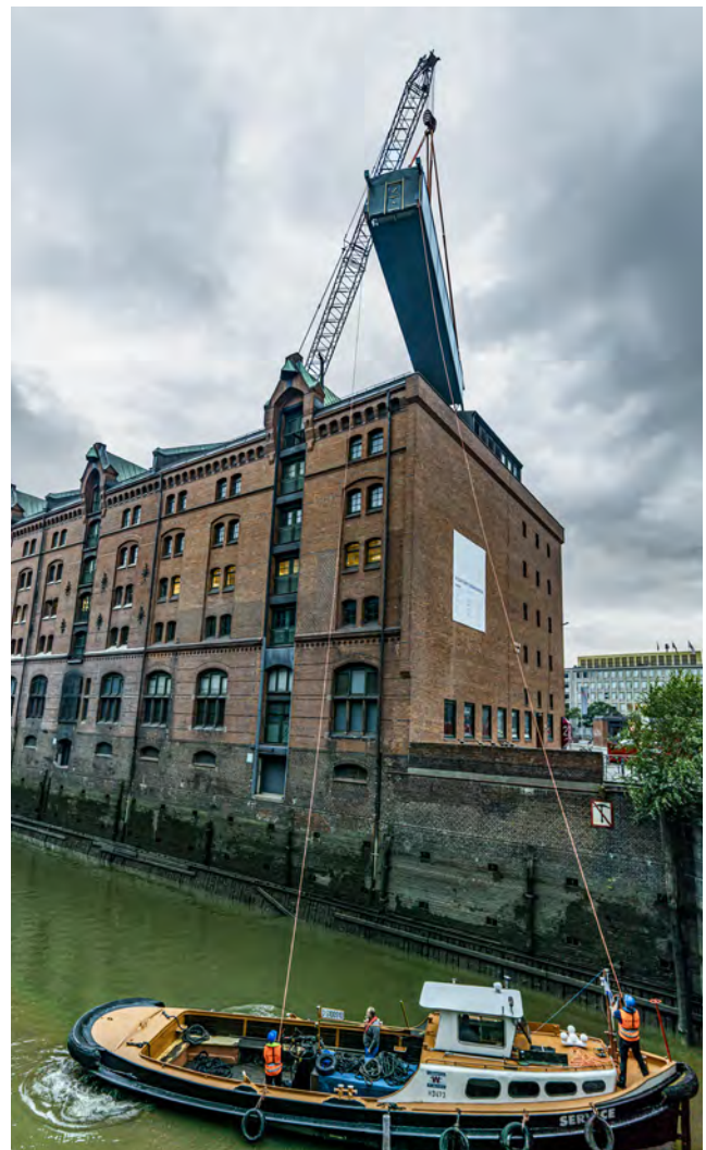
The retaining ropes are held on a small barge as the bridge is swung over the canal.
