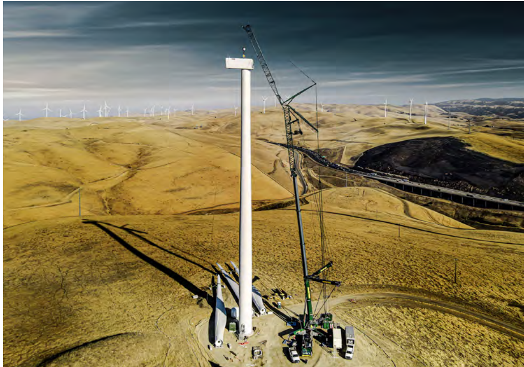
The 800 t upgrade made it possible to use the LTM 1750-9.1 at a wind farm in California.
