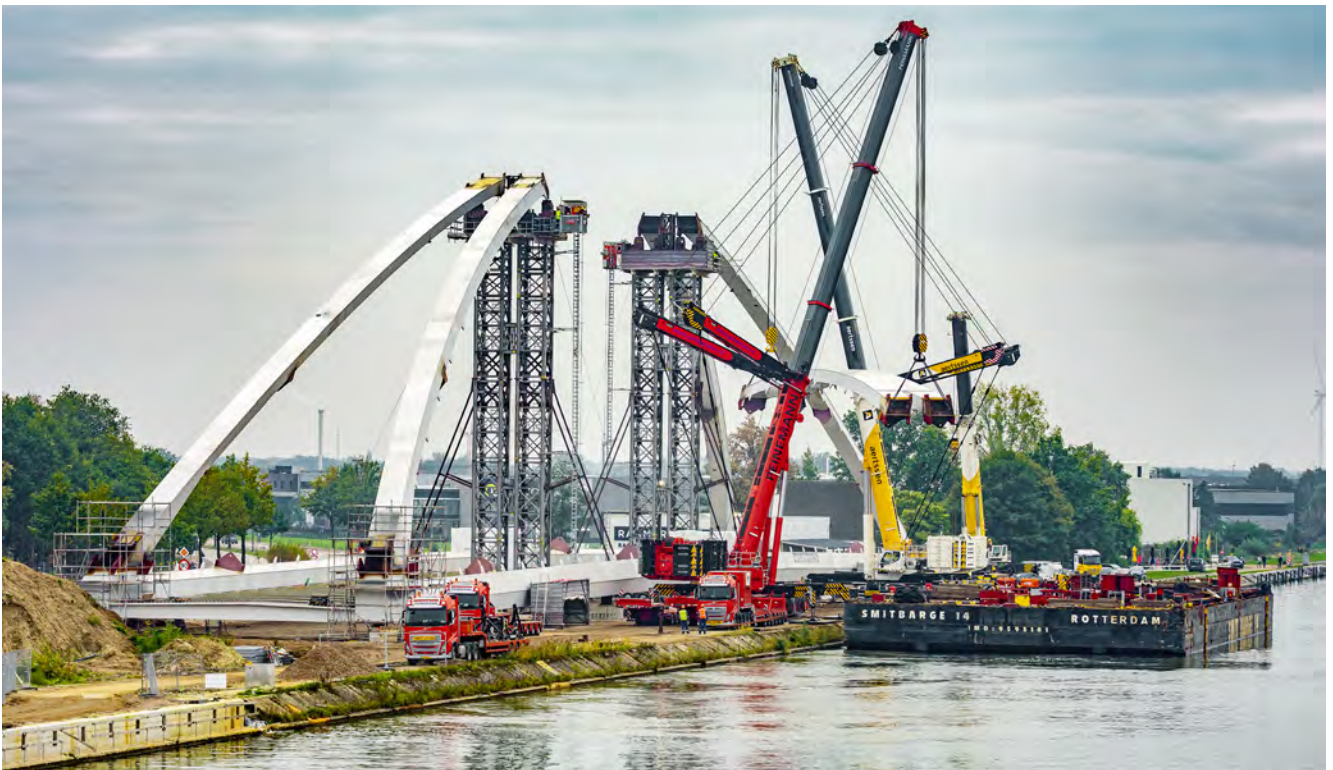
Guest appearance – many of the Dutch crane contractors are active throughout Europe or at least well beyond their own borders. Here you can see an LTM 1750-9.1 from Dutch contractor Peinemann giving a helping hand with the installation work for an arched bridge in Beringen, Belgium. The white and yellow Liebherr mobile crane of the same type is owned by Belgian group Aertssen.
