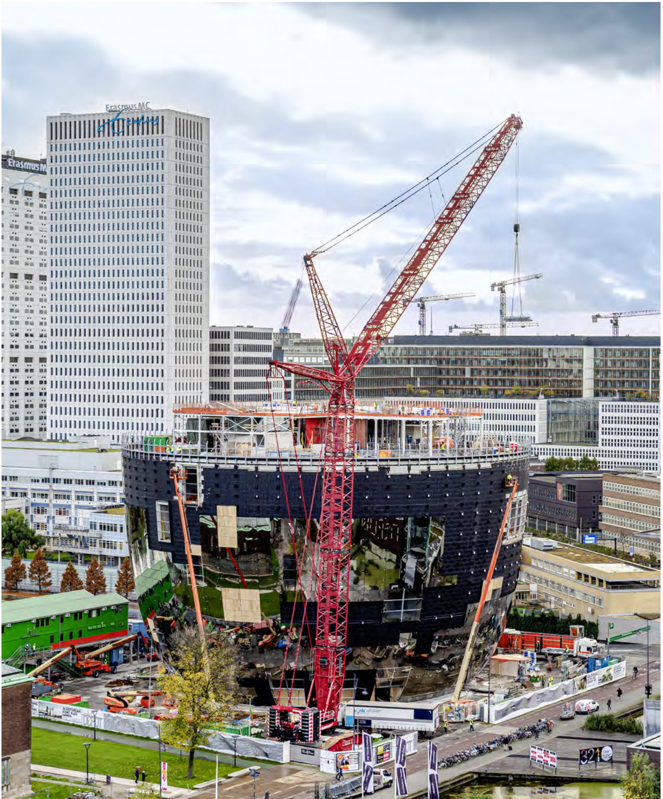
Futuristic – Mammoet's Liebherr LR 1500 crawler crane in action building a modern art depot for a museum in the centre of Rotterdam.
