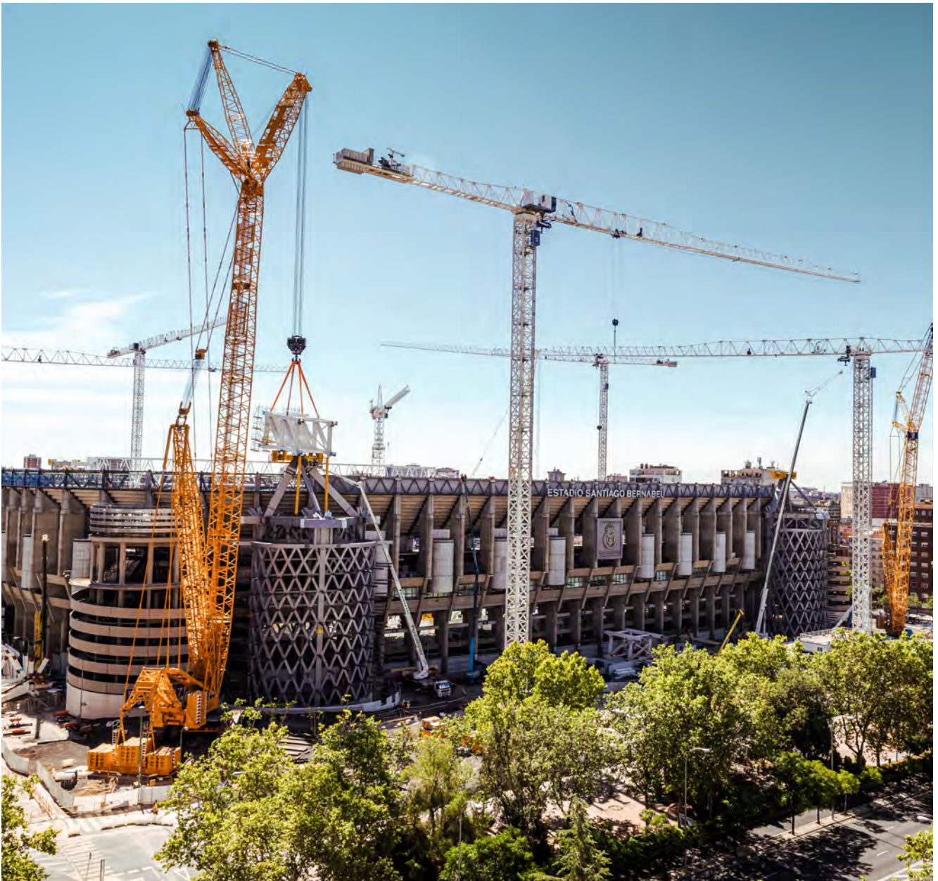
Playmaker – the LR 1800-1.0 from Eurogruas with some of the first segments for the roof supports on its hook.
