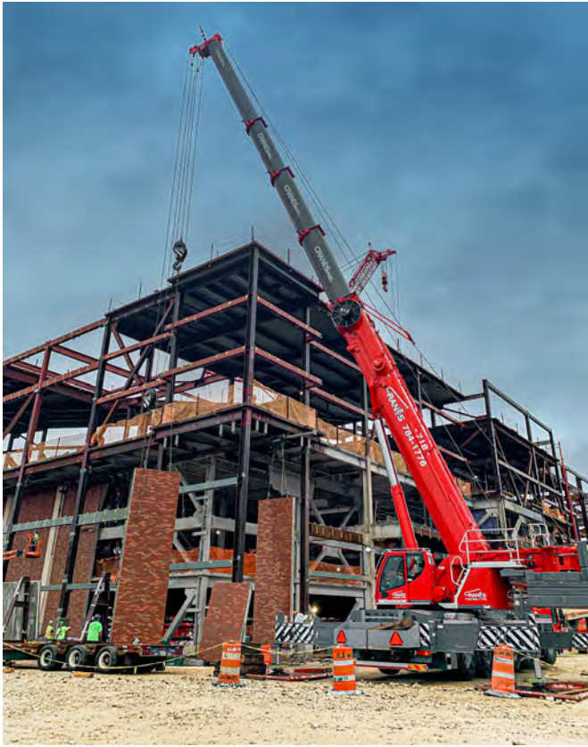
The LTM 1250-5.1 started in late June and just returned to the yard at the time of going to press.
