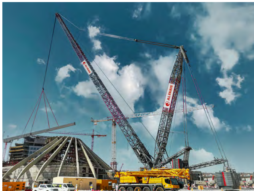
Al Faris erects 42 steel elements for the EXPO 2021 using the Liebherr LR 11000 crawler crane.
