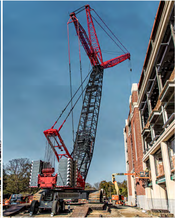
The LR 1500. Because the site is on the approach path to JFK International Airport, the maximum tip height is restricted to 73 m (240 ft.).
